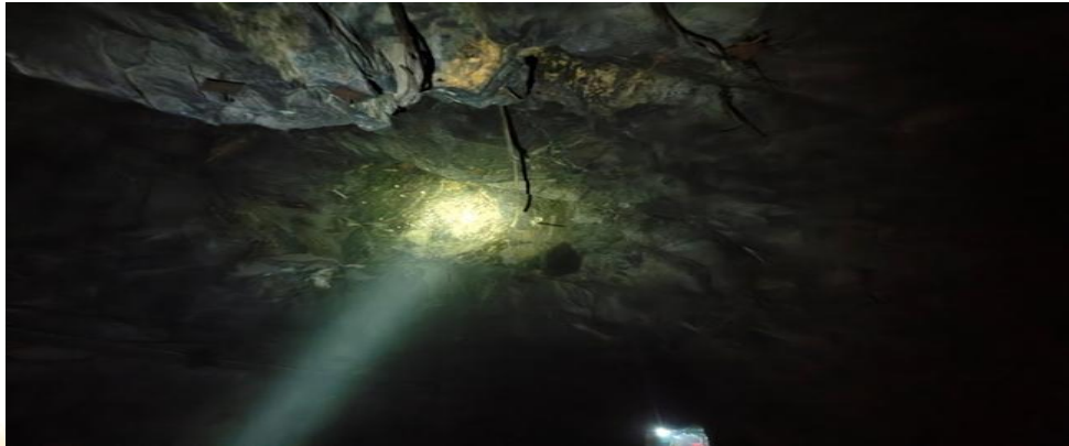
Fig. 5: Wedge failure observed at 89mRL decline drive.
