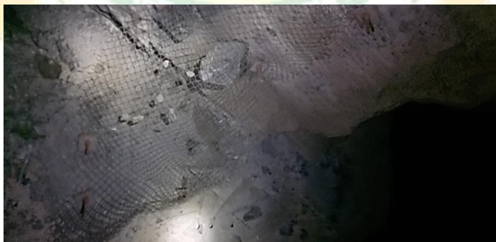
Fig.8: Roof condition near 14-16 VR at 120mRL.
